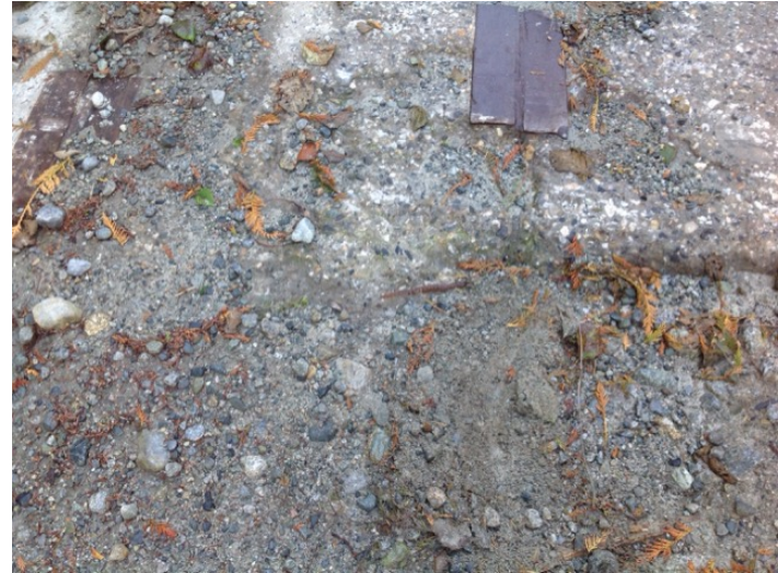
exposed rebar on slabs
